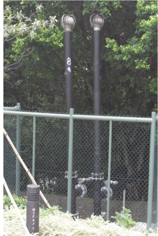
Photo 4 Landfill Gas Passive Vent Riser
