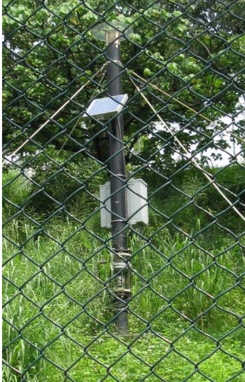
Photo 3 Solar Power Fan for Landfill Gas Venting System
