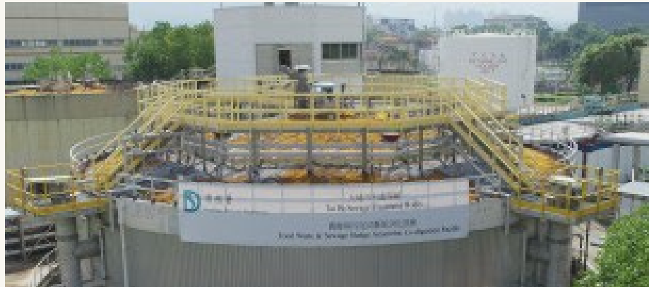
Food waste and sewage sludge anaerobic co-digestion facility at Tai Po Sewage Treatment Works
